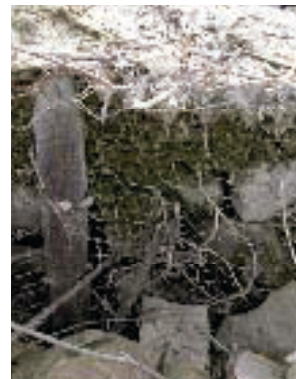
Figure 34. Example of a simple, cheap dam constructed with angled metal posts and galvanized wire in the channel of a small gully.
